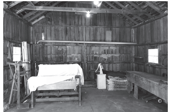
Debris was removed from the carriage house making ready for structural repairs
